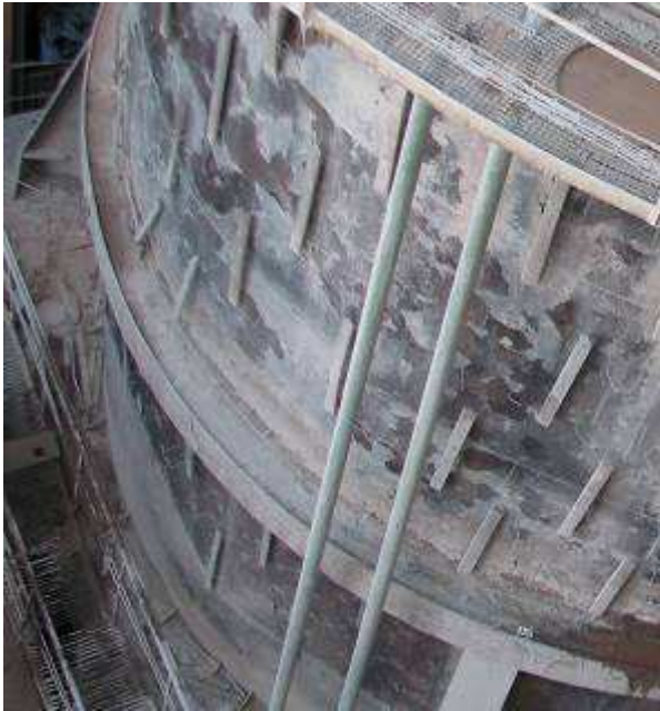
Figure 2. The damaged wall of the air conditioning tower between the fixation rings and above them
