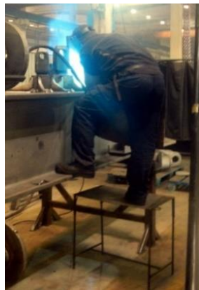
Fig. 3. Unsafe work situation
